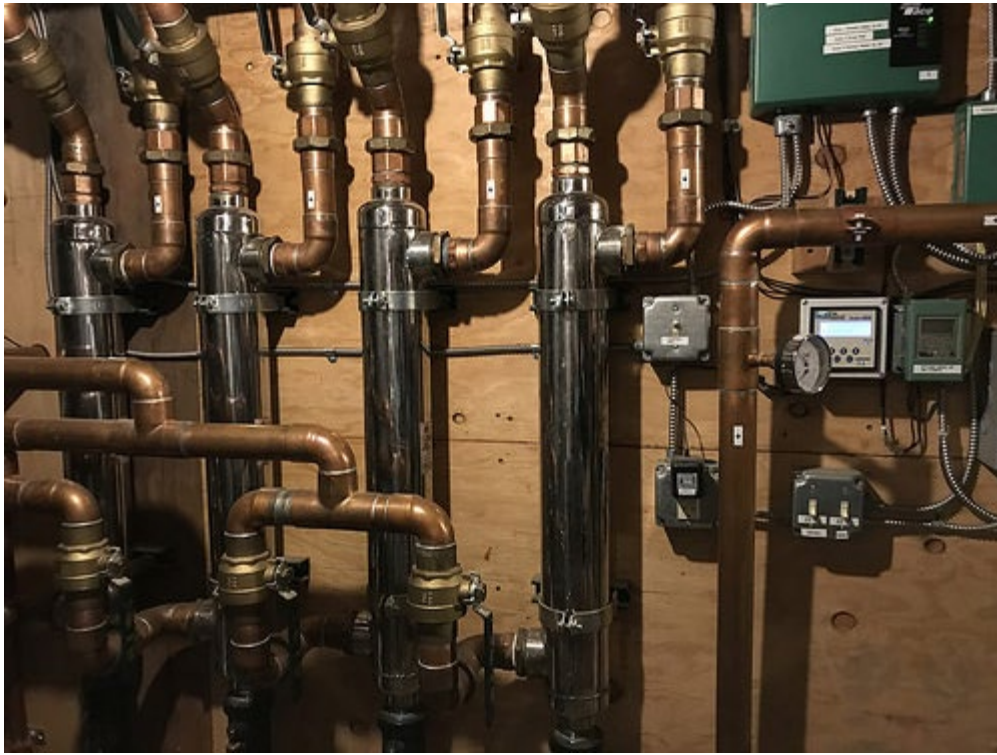
The Riff Raff Brewing Company Geothermal Mechanical Room
